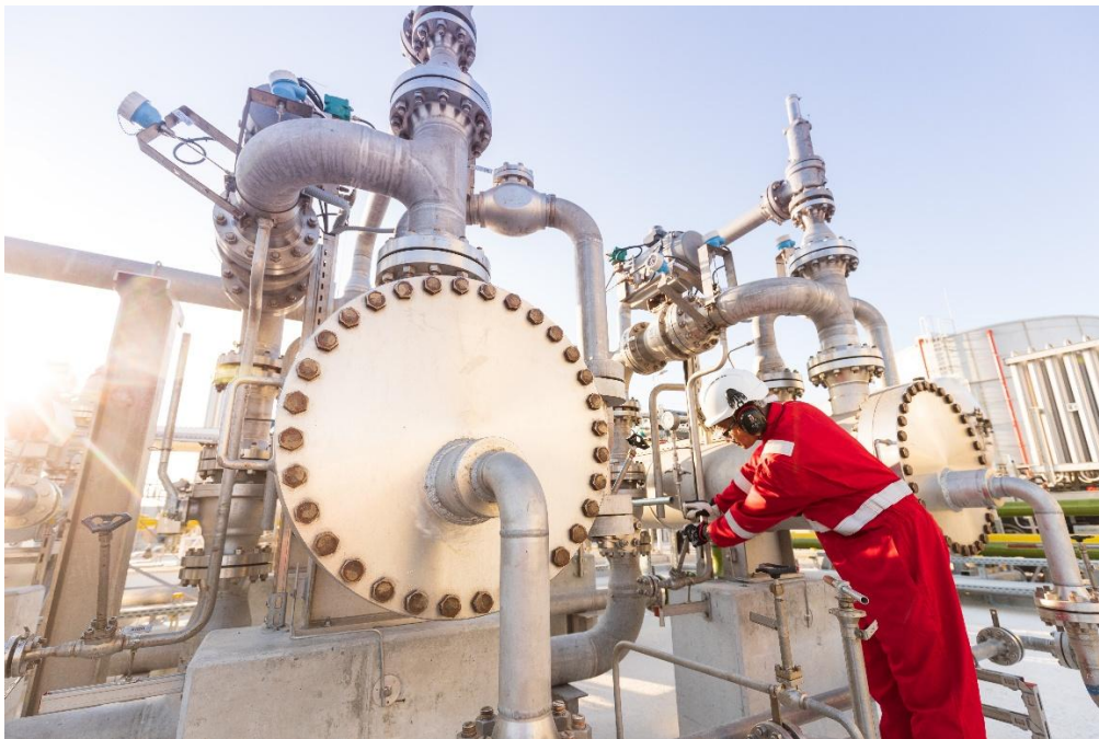
Shell's LNG regasification terminal in Gibraltar, which is switching from diesel-fired power generators to cleaner natural gas. A newly commissioned 80-megawatt gas-fired power plant will be used, Shell explains. An inspector checks the evaporator's gas pressure gauge. / Source: Stuart Conway / Shell
